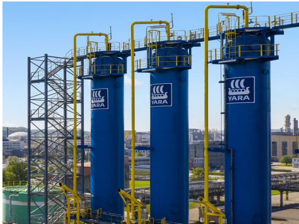
The green hydrogen demonstration plant will be the second 24-megawatt platinum-based electrolysis facility designed and constructed by Linde Engineering. Picture credit: Yara
